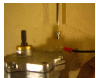
Feed Motor with Ground Wire.
