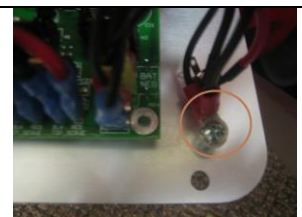
g. Ground wires from feed and battery negative black wire
