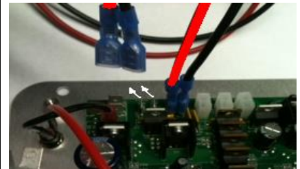
Top Server Motor wires (Red and Black) being unplugged.
