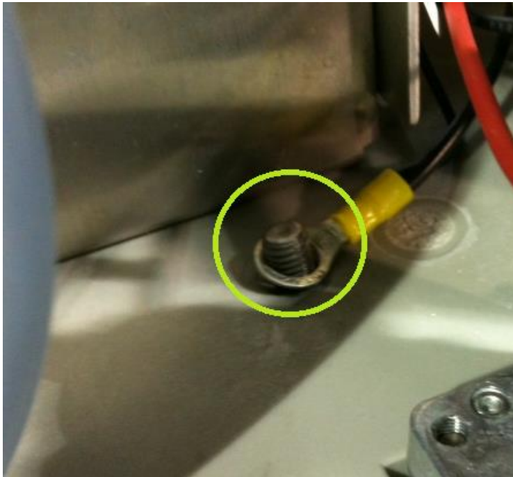
Bolt Nut (on inside of machine near bottom server wheel and sweep motor).
