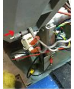
Ball Chute "Trap Door" pin being pushed to secure trap door.
