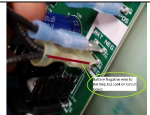
Battery negative connected to Bat Neg J12 on circuit board (marked in dark red).
