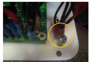
h. Ground Wires (marked in gold)
