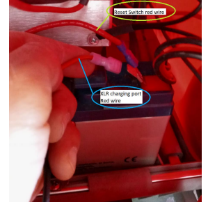
Red XLR wire, and Red reset switch wire to battery.
