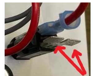
Reset Switch with terminal for red XLR charging wire, and Battery Positive wire coming from battery, marked by red
